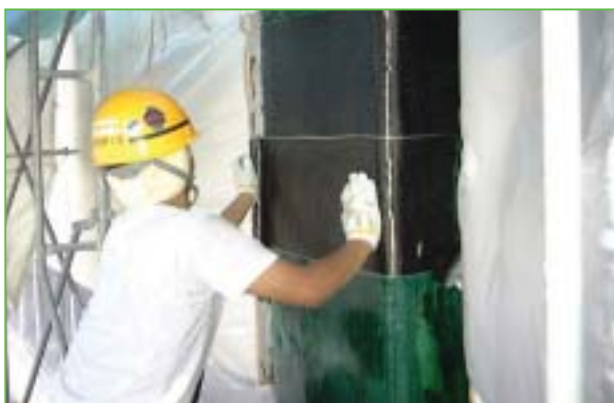
Earthquake proof construction in the Toyohashi Production Center
